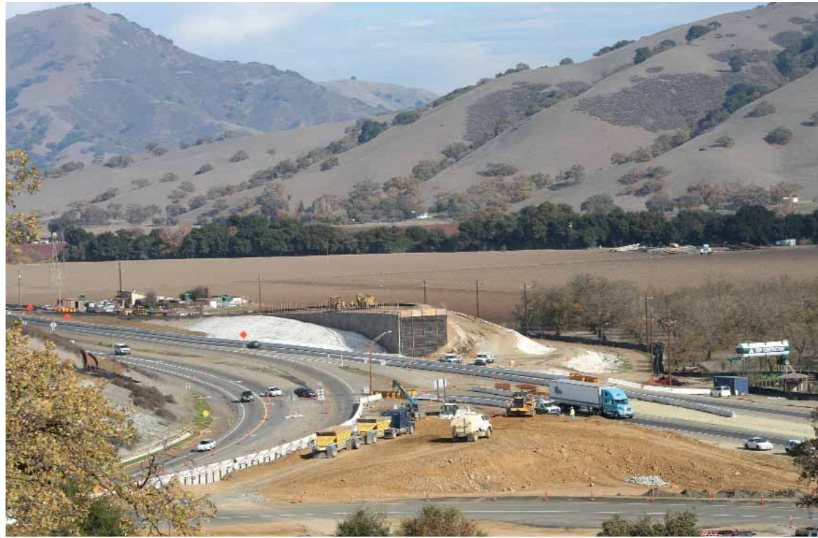
The Route 152/156 Improvement Project, from a hill just south of the project limits, shows the project in phase three. The office is located in the buildings in the distance, the north bridge approach is complete and the south bridge approach is under construction.
